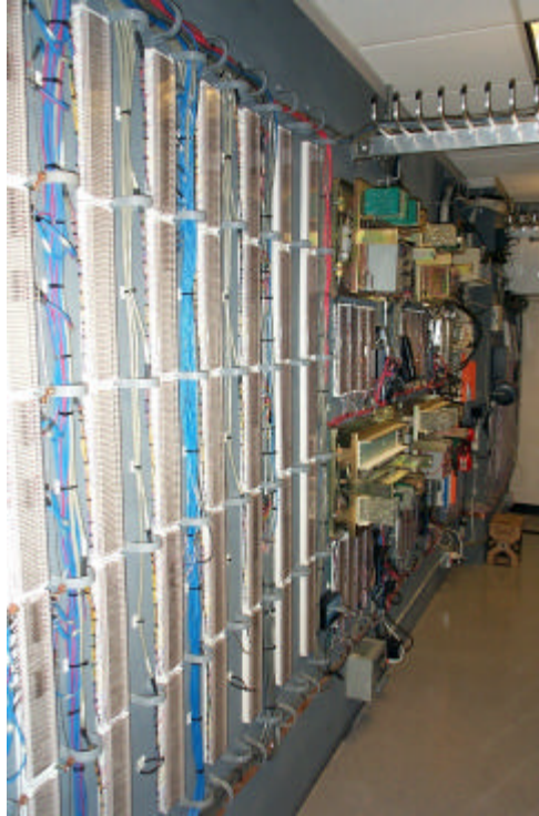
Wall of "66" punch blocks
