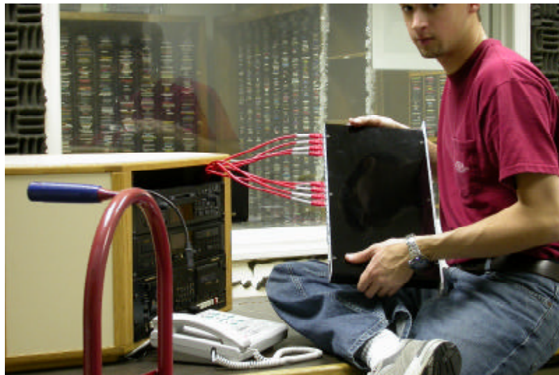
An analog audio node interfaces equipment in this rack to the network.
