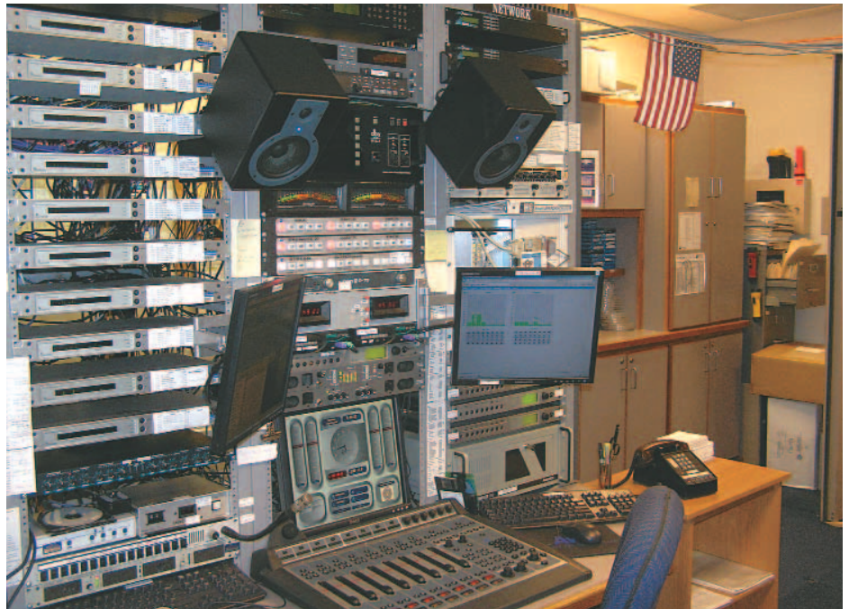
Journal Broadcast engineering rack following installation of Axia nodes.
