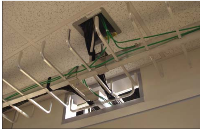
A wire tray exits the TOC feeding individual studios through square cable chase conduits.
